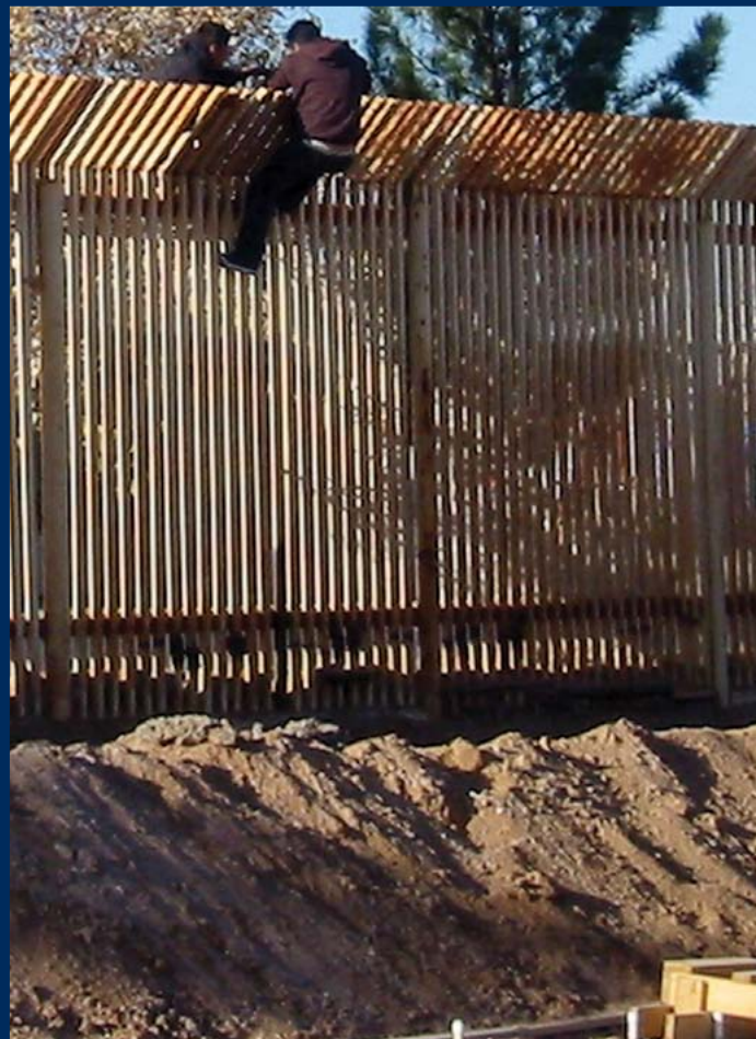
Two men scale the border fence between Mexico and Douglas, AZ, a few hundred yards away from where Seabees from Naval Mobile Construction Battalions (NMCB) 133 and NMCB-14 are building a 1,500 foot-long concrete-lined drainage ditch and a 10 foot-high wall to increase security along the US and Mexico border.
